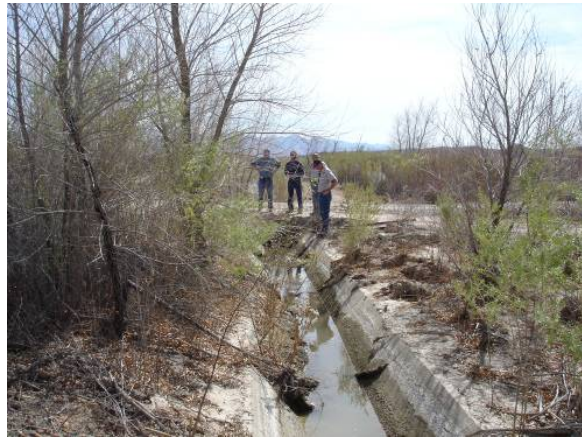
Figure B11d: Damaged water supply canal to Middle Pond.
