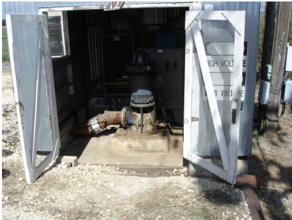
Figure B10c: Well house and power head for Burkett Well (to be refurbished).
